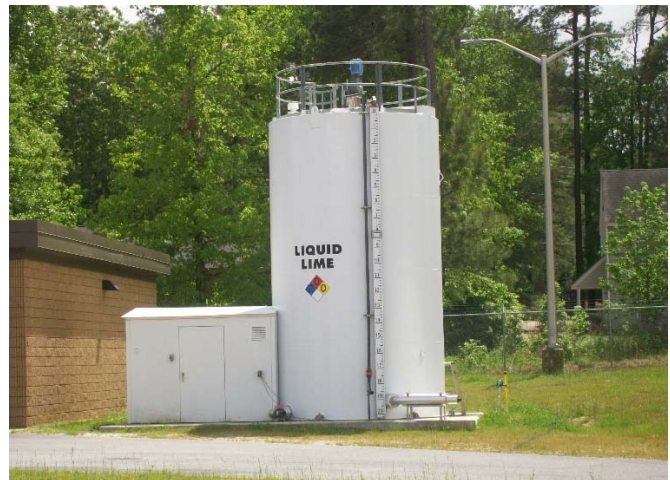
New lime tank and its chemical feed facilities
