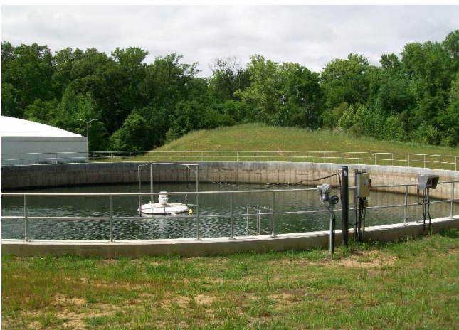
1.5 million gallon backwash storage tank
