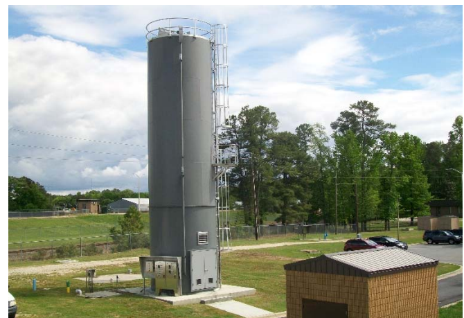
Powder Activated Carbon storage tower and feeder
