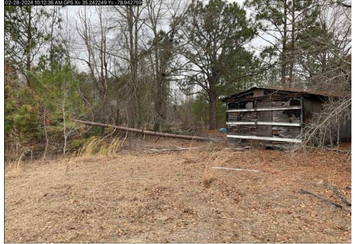
Site View Abandoned Structure
